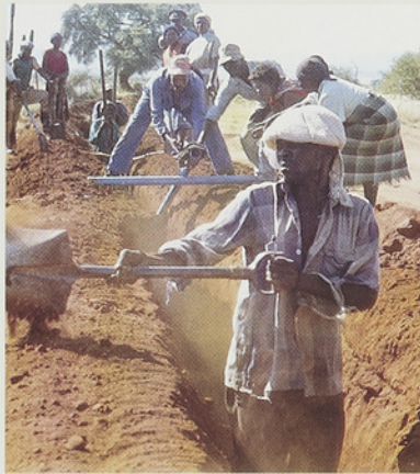
Villagers from Mabeskraal line trenches with soft soil to accommodate the trunk mains that will bring water to their village in arid northern Bophuthatswana.
